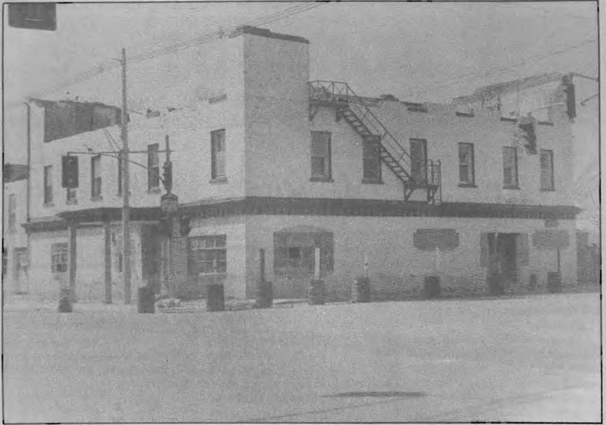
The Ingersoll Inn, a landmark in the town, is coming down. Workers with J & A Demolition and General Contractors of Tillsonburg are dismantling the structure. At left, is a view from King Street West, while
