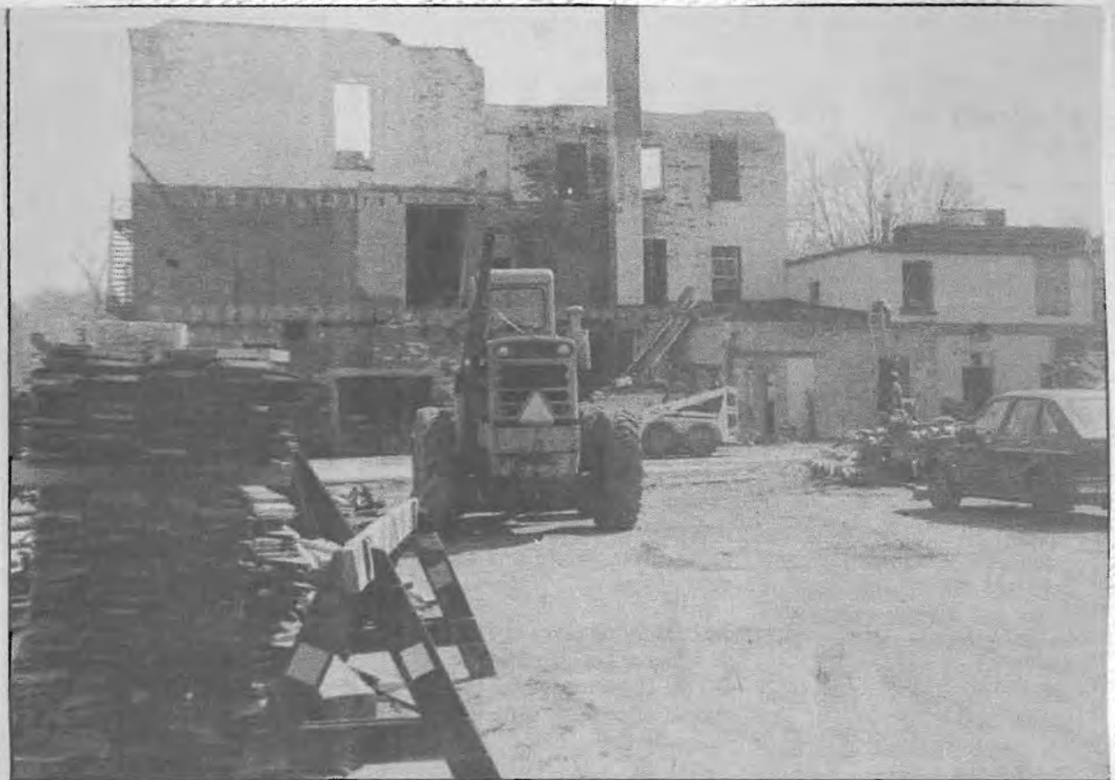
the photo at right shows the demolition from Oxford Street. (Liz Dadson photos)
