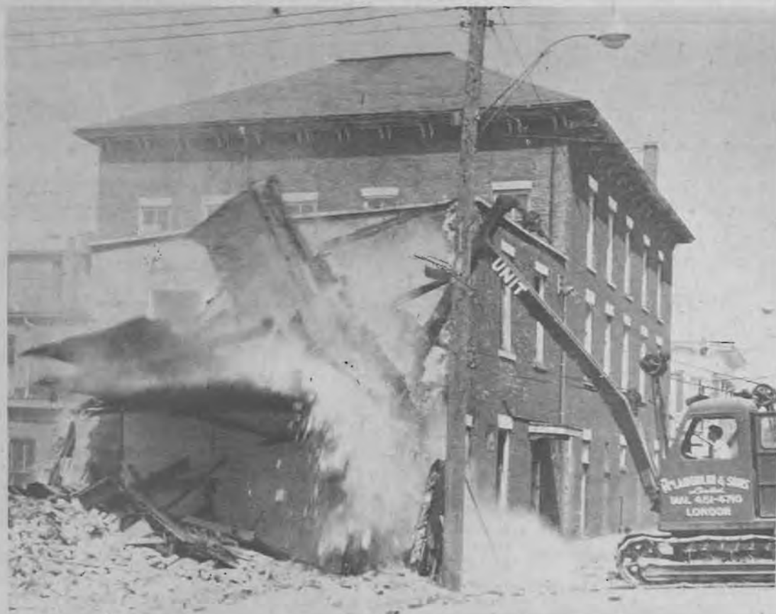
Demolition work of the rear portion of the St. Charles Hotel began last week in preparation for renovation of the main building. A modern hotel is planned for the site. Interest is keen on just what will be done to the old landmark.
